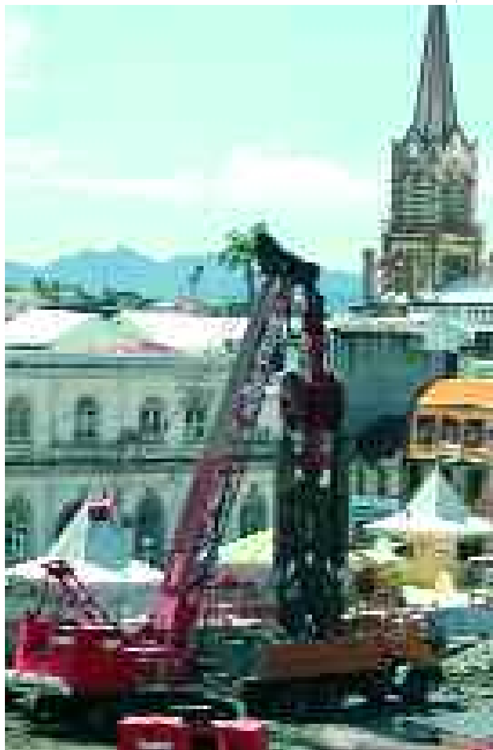
The Perrinon car-park is one of the largest foundation works projects in the West Indies.
